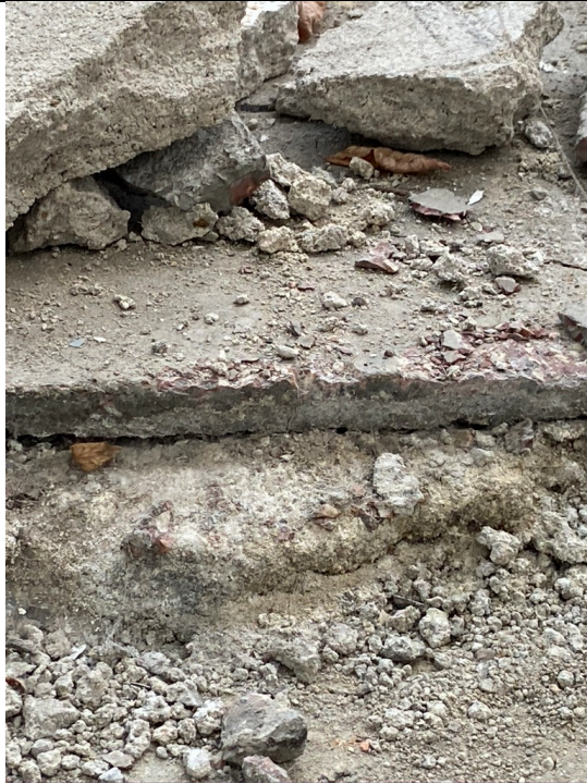
Spinning mill from approx. 1890, northern interior, broken edge of a machine pit: Under the destroyed recent concrete messenger, a possibly original slab of red terrazzo. Photo: Ivo Hammer 2021
