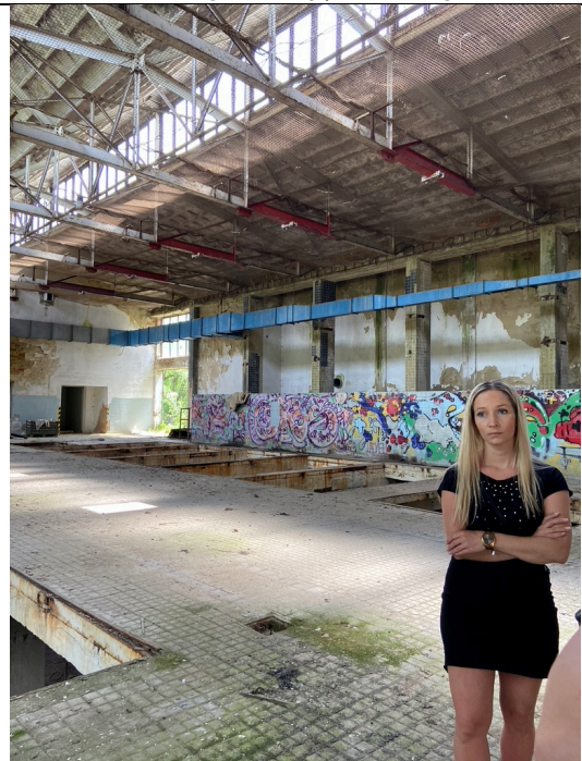
The walls are tiled up to the level of the sills of the north windows (blue, yellow, black). On the south side there is an additional tiled wall, probably as a splash guard (with recent wall paintings)
