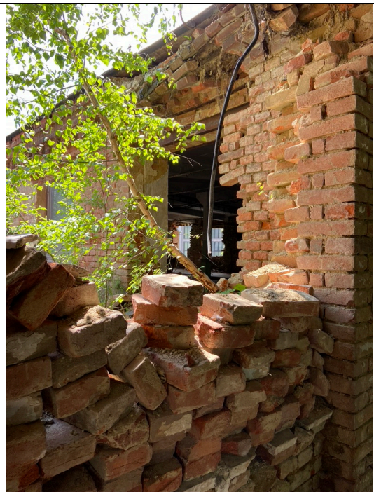
Schindler's Ark, 2nd floor, reinforced concrete hall, northern annex room, view to the southwest, detail. Photo: Ivo Hammer 2021
