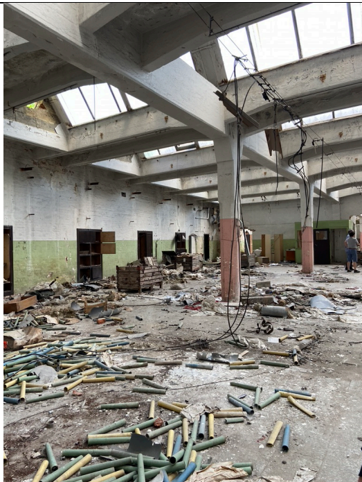
Spinning mill from approx. 1890, south interior, view to the northwest. Photo: Ivo Hammer 2021
