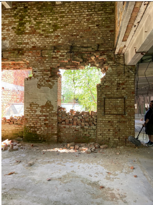
Schindler's Ark, 2nd floor, reinforced concrete hall, northern annex room, view to the south. Photo: Ivo Hammer 2021
