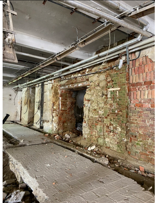
Schindler's Ark, ground floor, reinforced concrete hall, view to the northeast. Breakthrough through stone and brick wall. Bricking up a window. Photos: Ivo Hammer 2021
