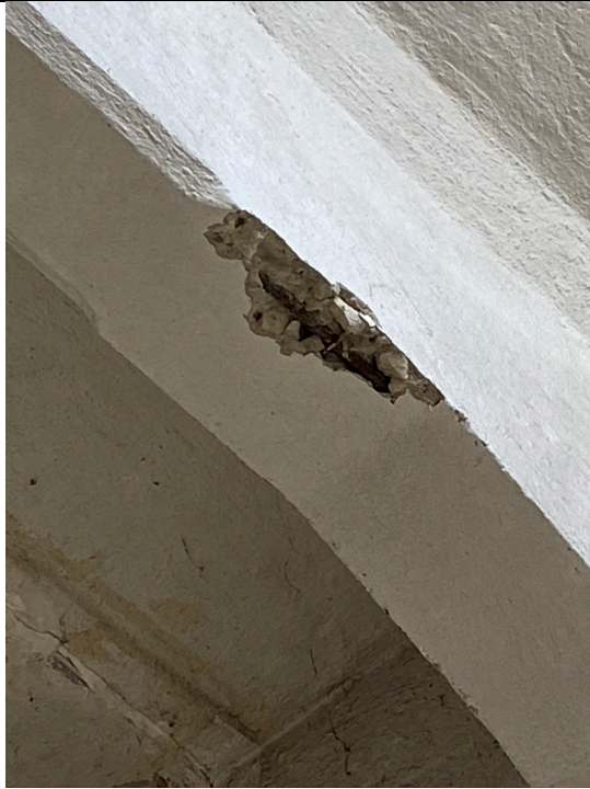
Spinning mill from approx. 1890, northern (?) Interior, detail of a cross member. The gray cement mortar and the reinforcing iron are visible in the mechanical damage. Photo: Ivo Hammer 2021
