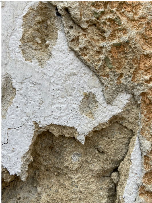
Residential building (management by Oskar and Emilie Schindler), facade detail: base plaster with yellowish-gray mortar with fine lime sparrows (dry slaking), fine plaster with the same mortar, only finer grain size.
