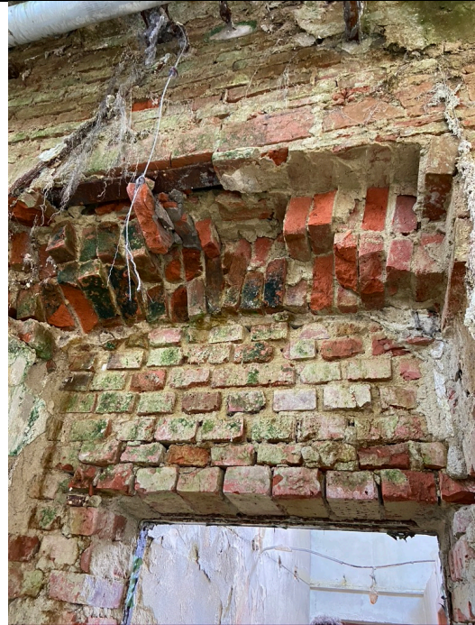
Spinning mill from around 1890, northern interior, east wall, detail. The brownish masonry mortar is visible on the broken-out segmental arch overlay of the door. Photo: Ivo Hammer 2021
