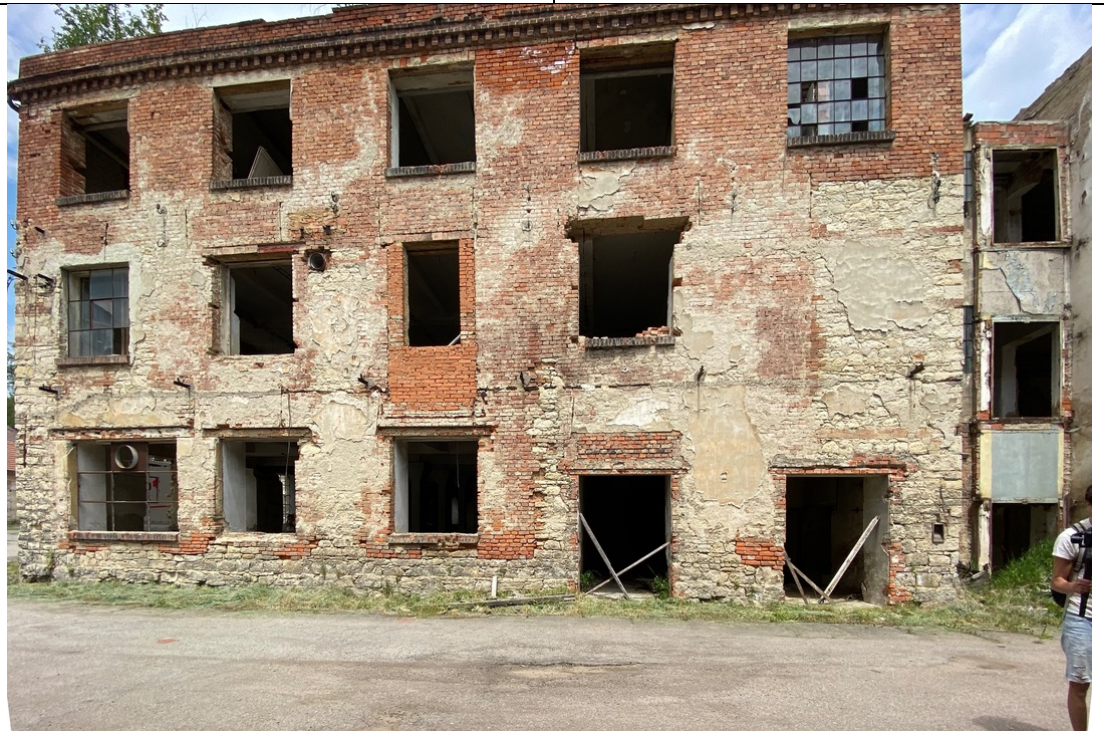
Brnenec, Schindler's Ark, south facade. On the east facade, a secondary staircase is installed in the space between the adjoining building. Rebuilt several times.
