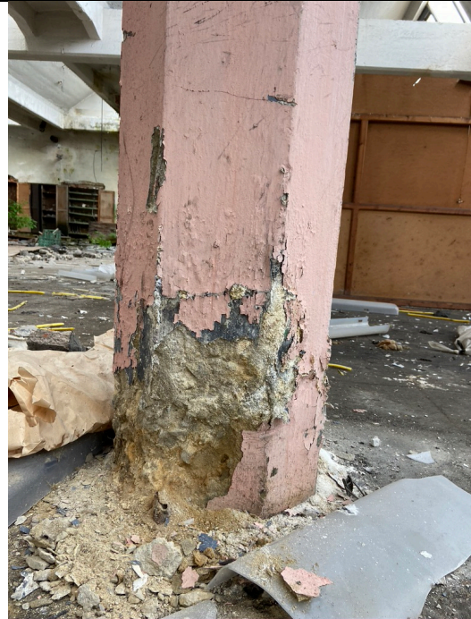
Spinning mill from approx. 1890, south interior, detail of a pillar. The cement is the brownish Roman cement. A touch up? Photo: Ivo Hammer 2021
