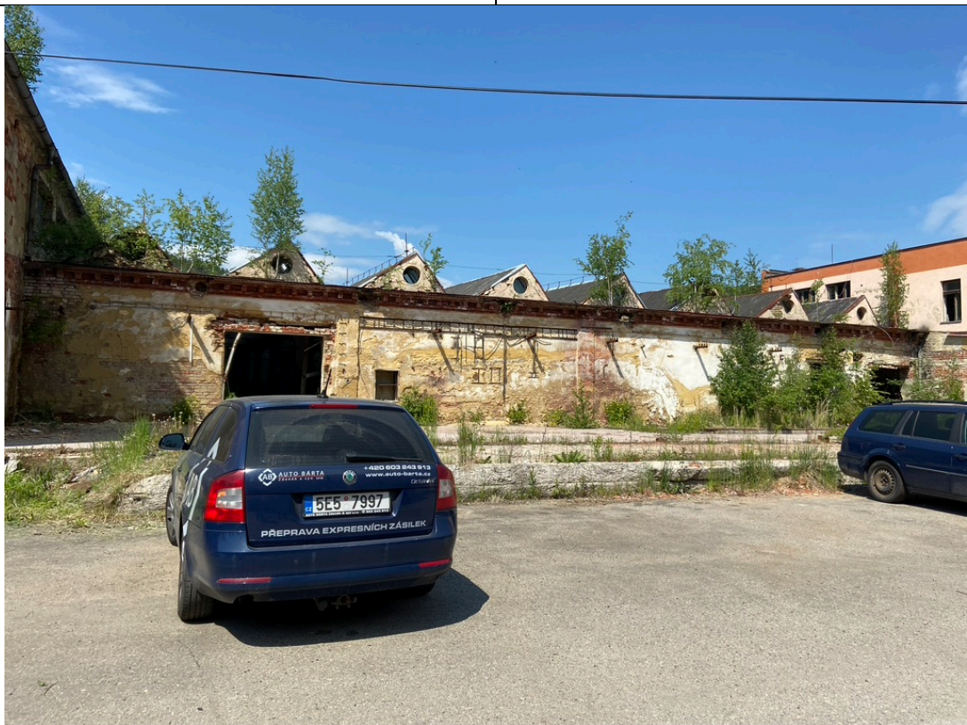
Spinning mill from approx. 1890, outer facade of the southernmost part, the later) vestibule has been removed; Structure of the smooth plastered façade with pilaster strips and serrated eaves made of brick, originally presumably yellowish-white lime paint, later several whitewashes in yellow and pink. The oculi of the hypetheral roof are bordered with fascia. The eaves of the roof gable may have originally only been protected with sheet metal. Photo: Ivo Hammer 2021
