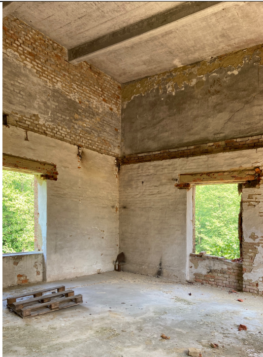
Schindler's Ark, 2nd floor, reinforced concrete hall, northern annex room, view to the northeast. Photo: Ivo Hammer 2021
