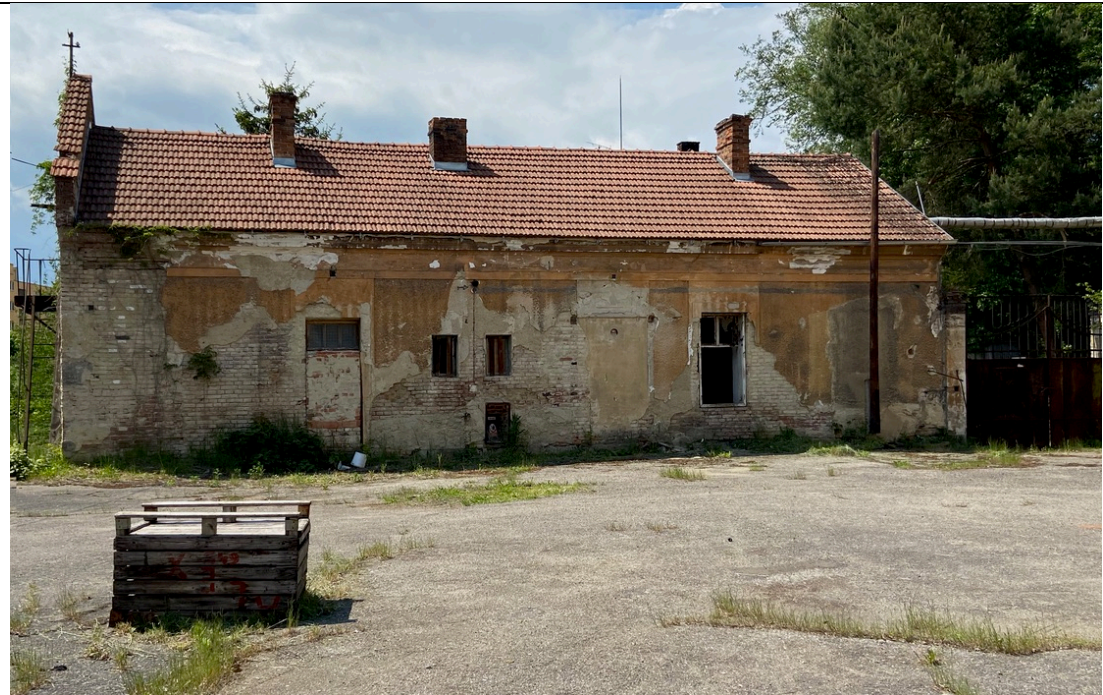
Residential building (management by Oskar and Emilie Schindler). Brick, block bond. Profiled eaves cornice. Raised south gable. 3 (?) Chimneys. Walled up doors. A window walled up with cement mortar. Photos: Ivo Hammer 2021
