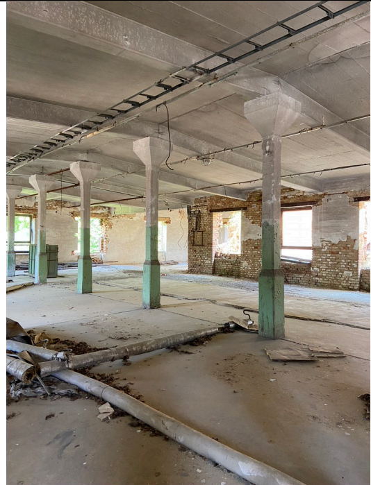
Schindler's Ark, 2nd floor, reinforced concrete hall, view to the northeast. Photo: Ivo Hammer 2021
