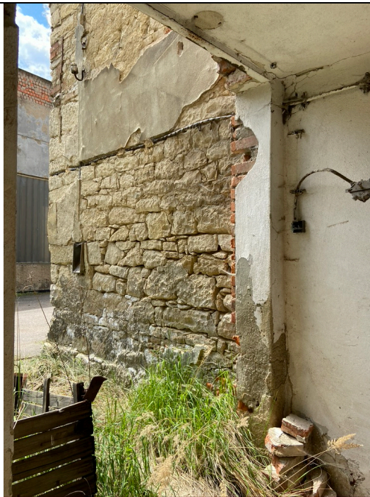
Schindler's Ark, east wall, detail of the south-east corner: stone masonry, sloping base
