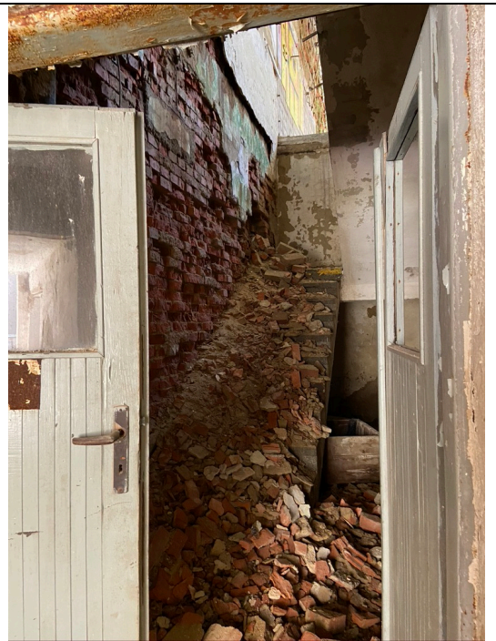
Space between Schindler's Ark and the annex to the dye works: concrete stairs. Photos: Ivo Hammer 2021
