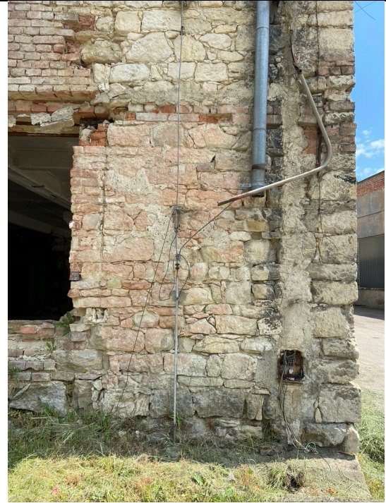
Local pink discoloration of the stone from the source of the fire.
