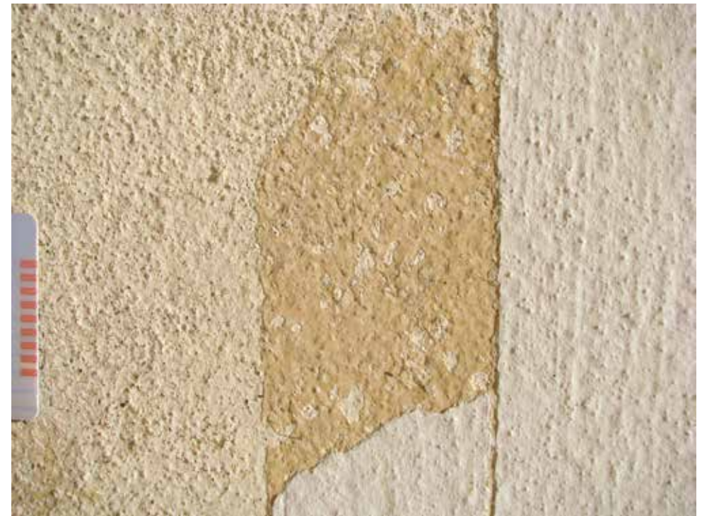
Brno, Tugendhat House upper terrace, east facade, probe paint layers; left: original surface, middle: two weathered lime washes, right: paint of 1985 containing resin
