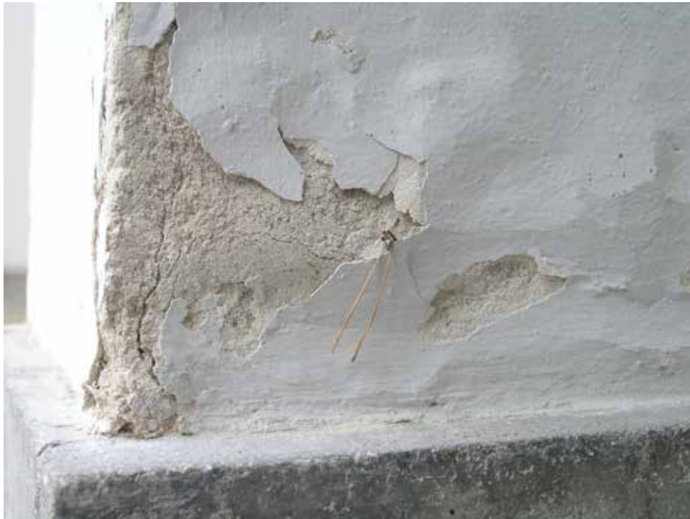
Dessau, master house Kandisky/Klee detail of facade, damages caused by incompatible coating materials from 2000 Photo: Ivo Hammer 2006
