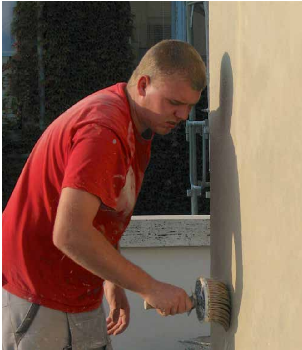
Brno, Tugendhat House upper terrace, south-west facade, artisan painting a lime wash prepared by conservators-restorers. Photo: Ivo Hammer 2011
